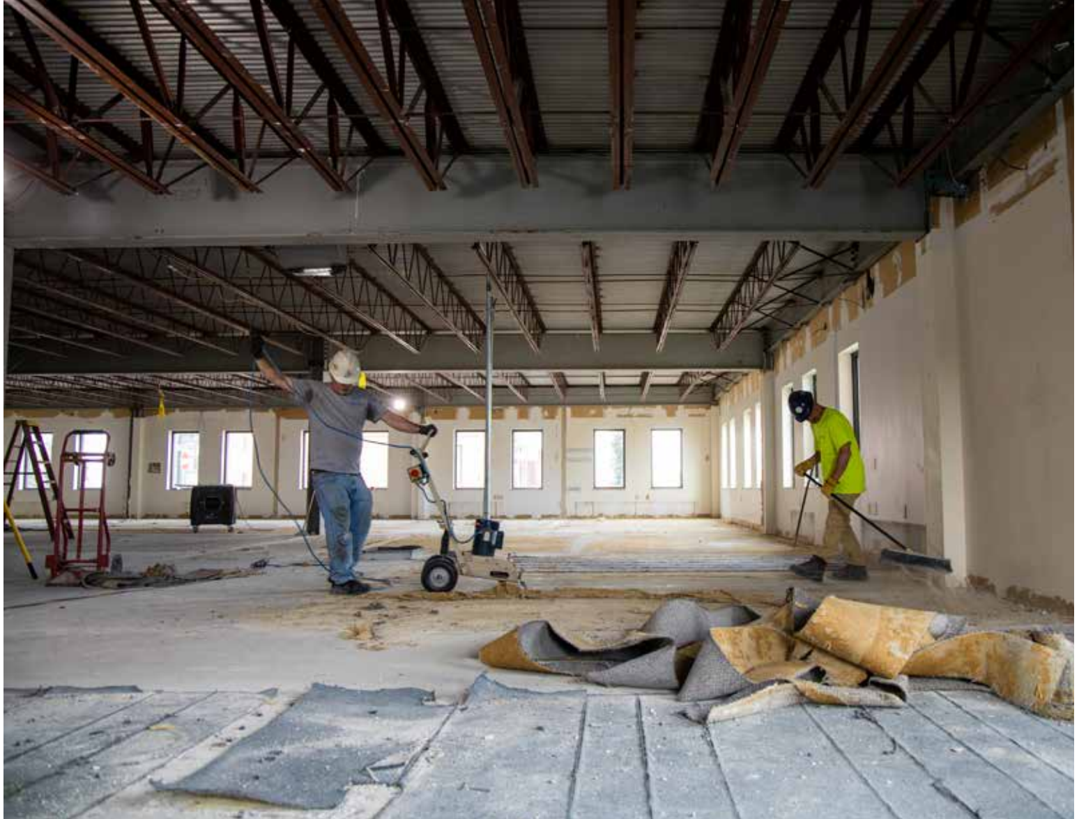
Renovations are underway at the future home of the Preble Street Healing Center to provide comprehensive services and case management for survivors of human trafficking in a dedicated safe space.
